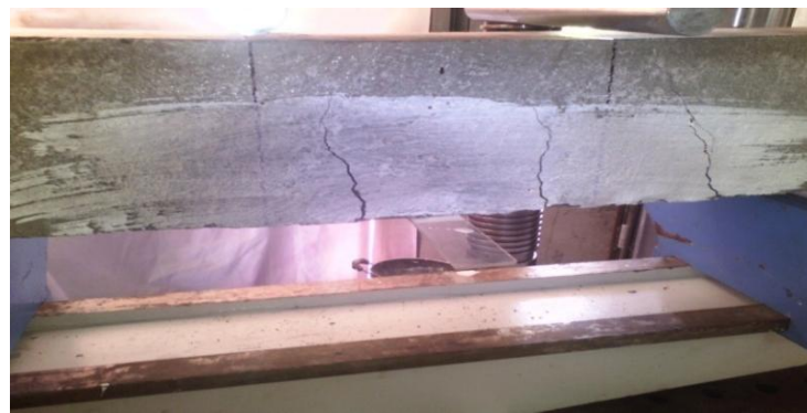
Figure.12 - Crack Pattern of the Beam Specimen
